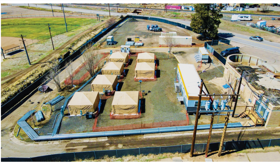
The South Railroad Facility shelter. Photo courtesy of the City of Loveland.
